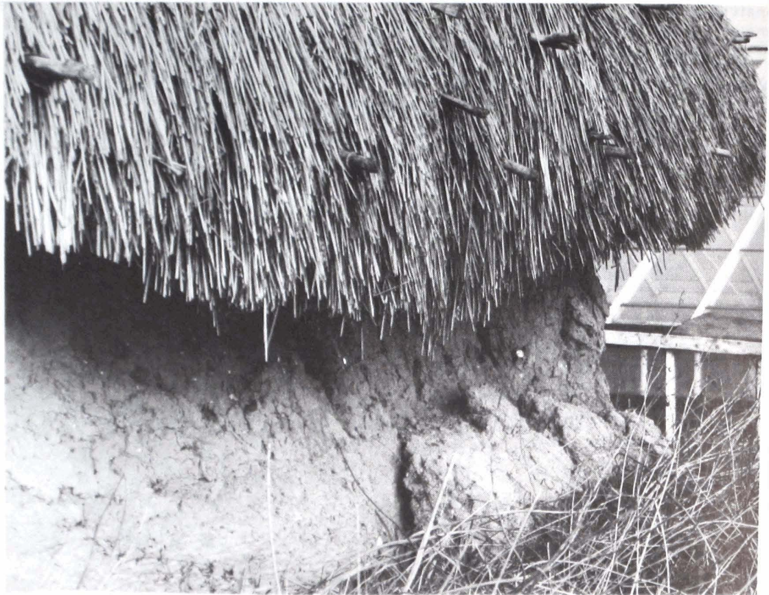
FIG. 4a. The high water table at Theobald's Park Farm barn has caused the soil walls to slump.
