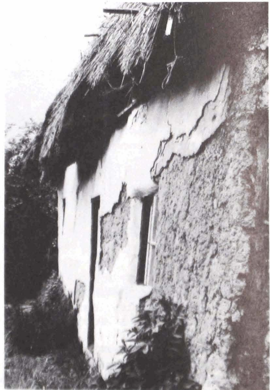
FIG. 4b. Animal infestation and salt efflorescing has caused surface spalling at Bedehouse Bank Cottage, Bourne.
